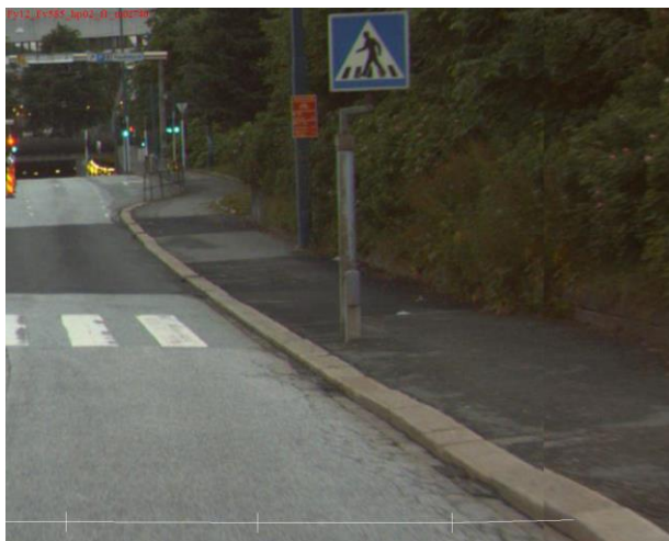
Figur 6.1: Krakelering inn mot fortau Hp 2 m 2740
